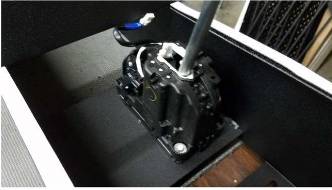
FIG 8 - SHIFTER INSTALLED IN CONSOLE
